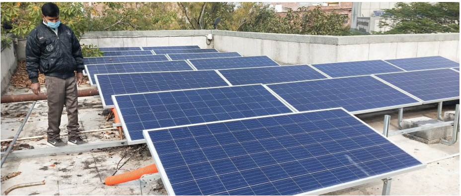
Figure 13: 36kW Rooftop solar system at RPVV, Hari Nagar.
